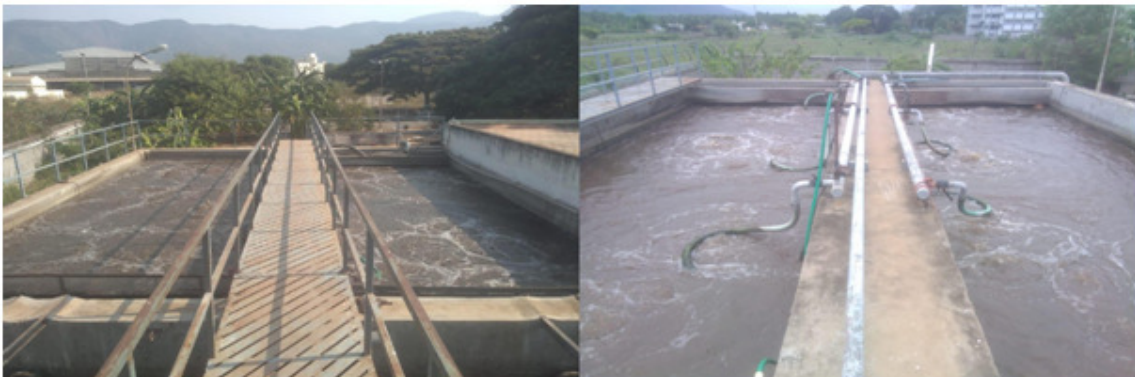
Figure 18. JMR and LH STP – aeration tanks
