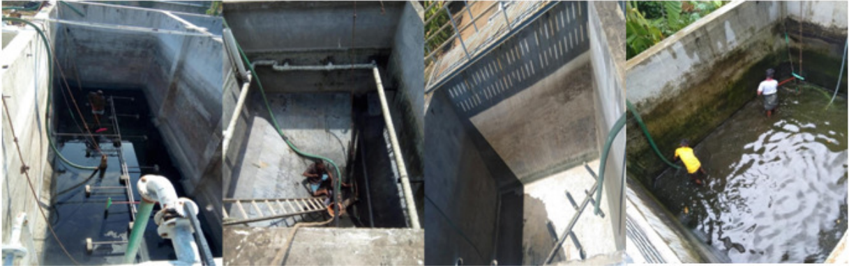
Figure 22. LH STP Cleaning – Collection tank, settling tank, filtered water tank and recycled water storage tank
