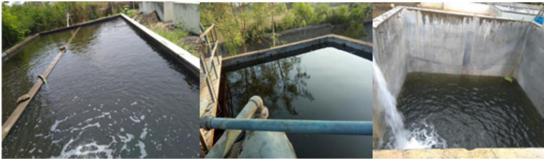
Figure 17. Storage tanks for treated water (before reuse in the garden)
