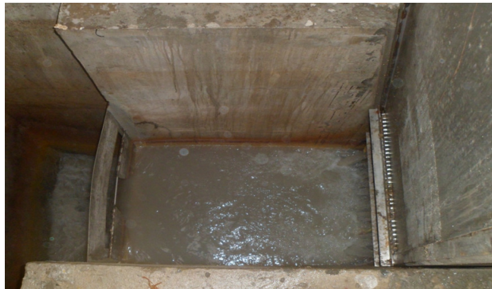
Figure 12. Sludge drying bed
