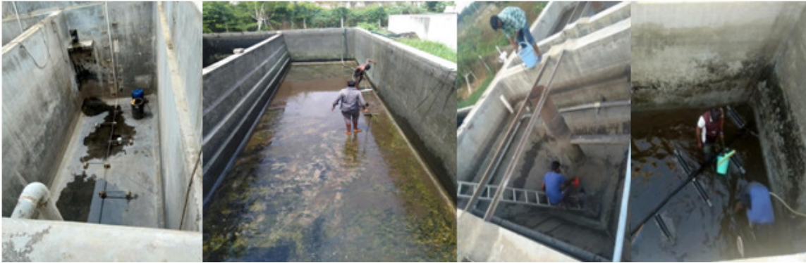
Figure 20. JMR STP cleaning – Collection tank, settling tank, filtered water tank and reuse water storage tank
