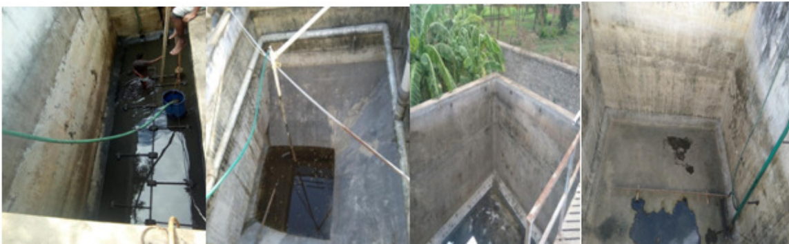
Figure 21 FDR STP Cleaning – Collection tank, settling tank, filtered water tank and reuse water storage tank
