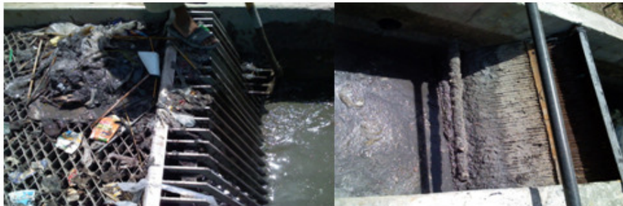
Figure 8. Primary screening unit
