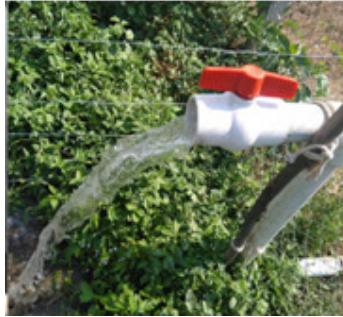
Figure 19. Outlet for the recycled wastewater from STP
