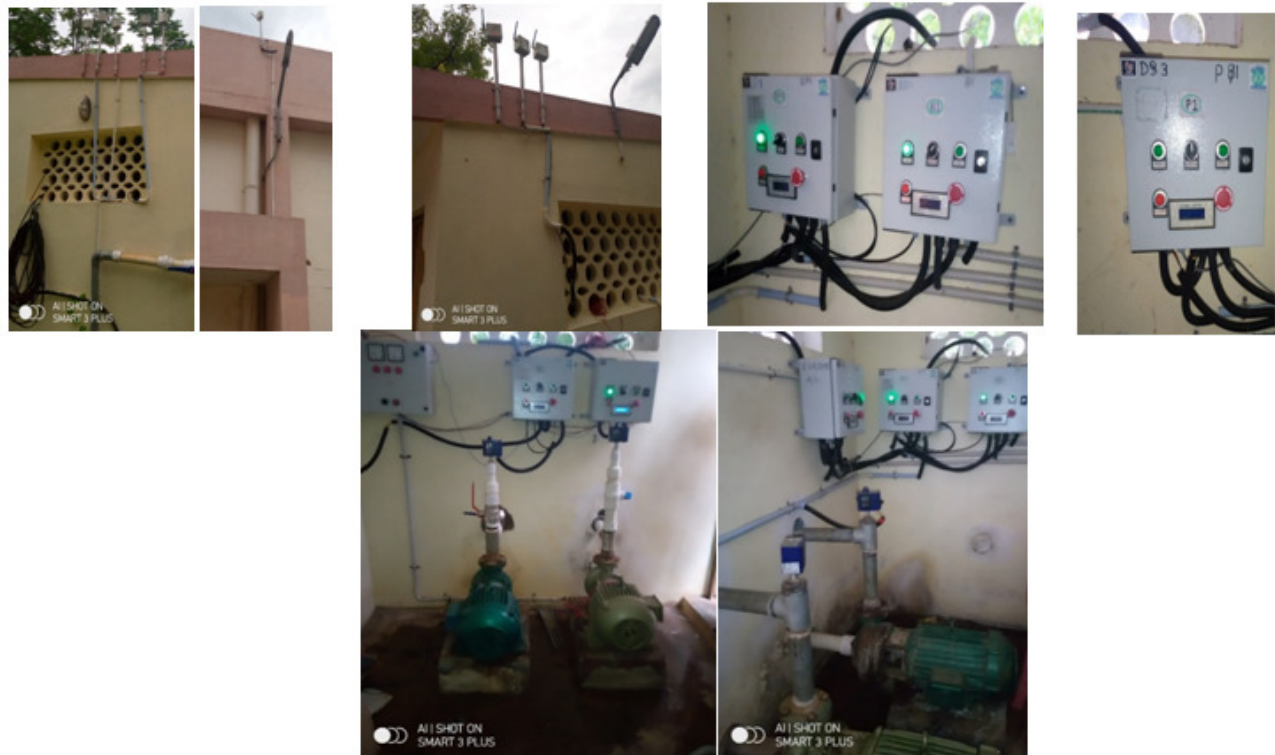
Figure 5 Automatic Waterflow Control Units
