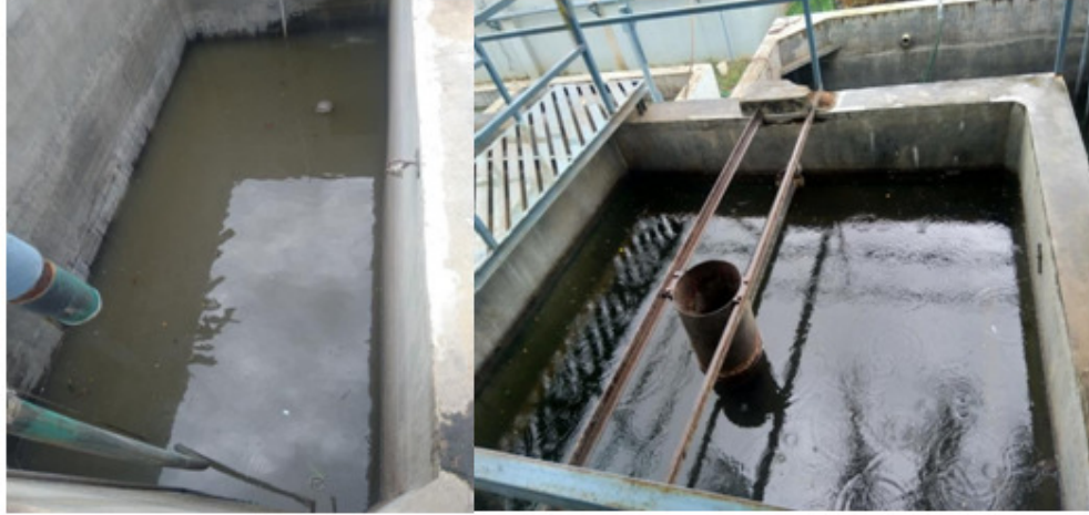
Figure 16. PRG collection tank, settling tank
