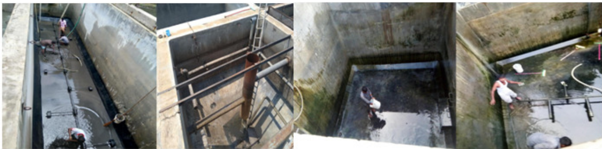
Figure 23. PRG STP CLEANING – Collection tank, settling tank, filtered water tank and reuse water storage tank
